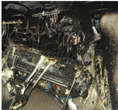
Fig 1. Consumer unit with plastic enclosure after a fire caused by a loose neutral termination
