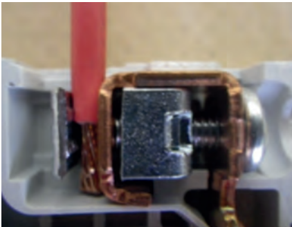
Fig 4. Termination made incorrectly as a result of insulation being trapped in the terminal clamp
