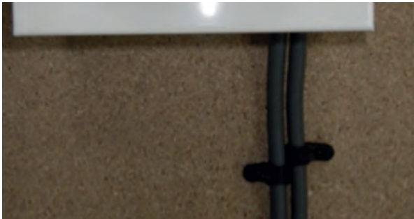
Fig 18. Meter tails secured by clips external to the consumer unit
