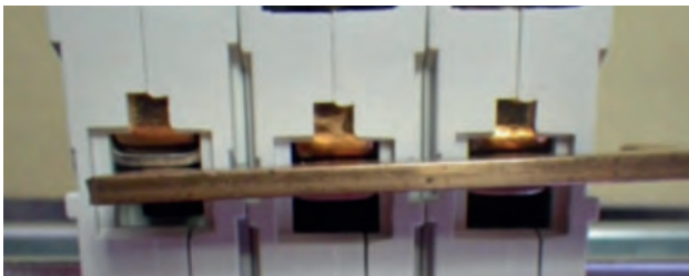
Fig 13. Circuit-breaker on left-hand side incorrectly installed with busbar tang/finger outside the termination clamp
