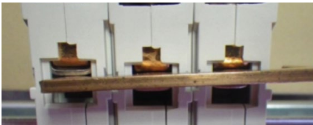
Fig 13. Circuit-breaker on left-hand side incorrectly installed with busbar tang/finger outside the termination clamp
