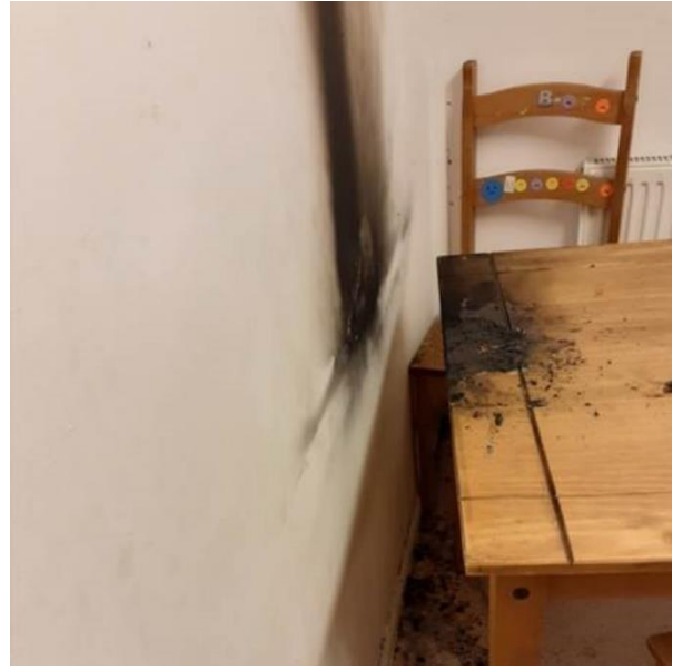
Damage to Rachel's property from the fire.
