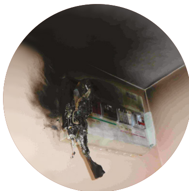
Result of DIY work by a home owner where a 10.5 kW electric shower was connected to a 45 A circuit-breaker using 2.5 mm 2 cable. (Photo courtesy of British Gas)
