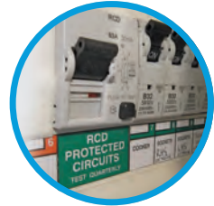
Fusebox incorporating an RCD.
